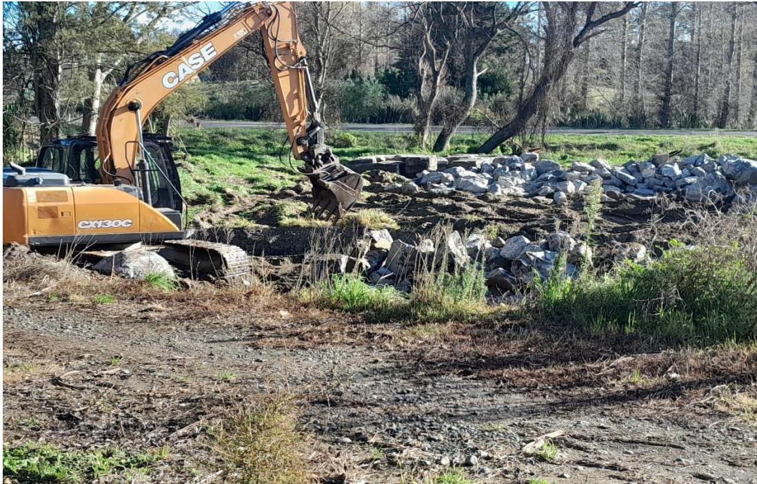
Diggers. Willows on stream bank removed. Dropping stream banks and inserting low rock wall to enhance channels 20 meters downstream.
